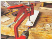
Drilling the support pillars for the dowel joints to attach them to the base unit
